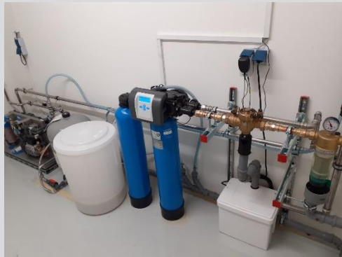
Water Preparation Unit
