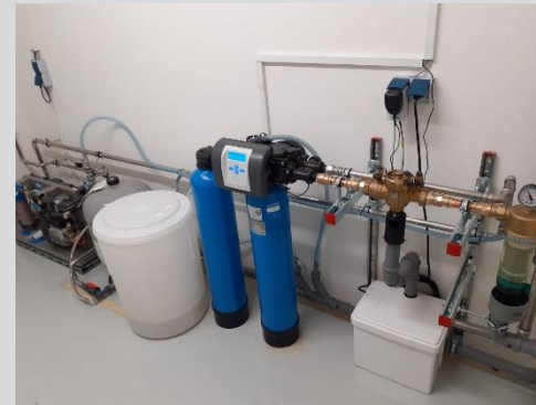
Water Preparation Unit
