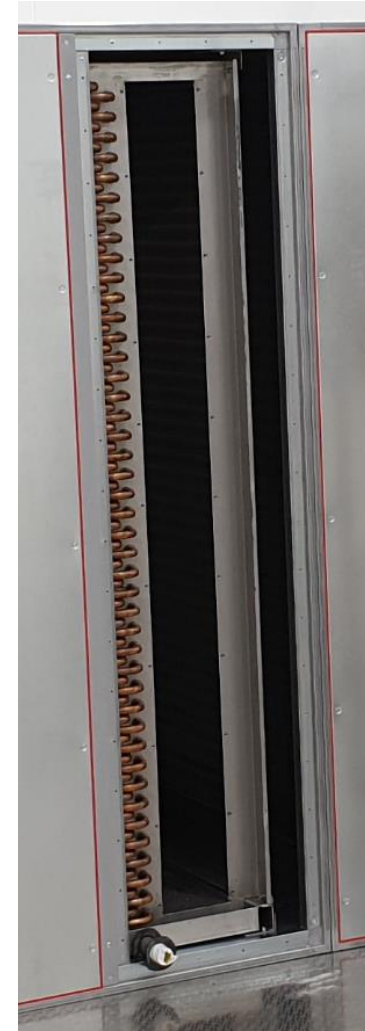
Heat Exchanger Unit installed in RLT with Drift Eliminator removed
